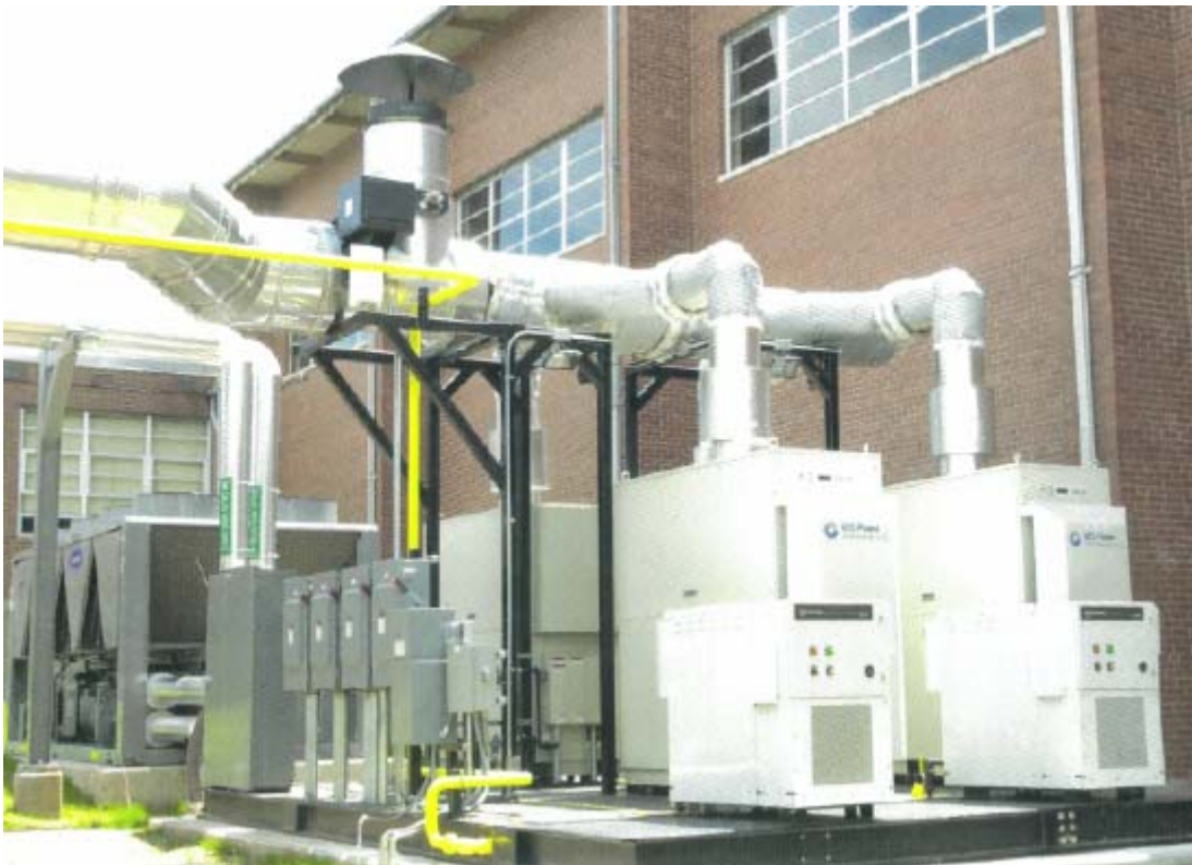
Figure 4: Outdoor installation of Pure Comfort Model 240 M
